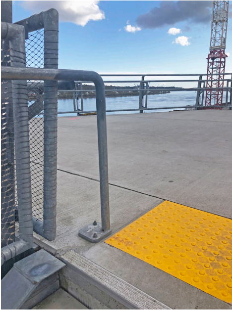
Example of tactile wayfinding surface indicator at the top of stairs (see policy 5)
