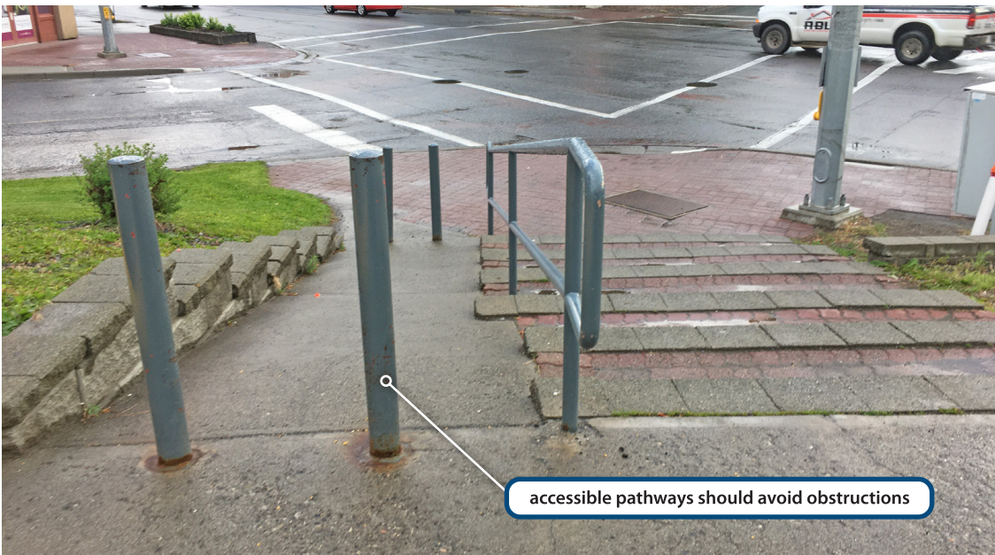
Accessible pathways should be a minimum of 1.5 m wide with no obstructions and achieve gentle inclines
