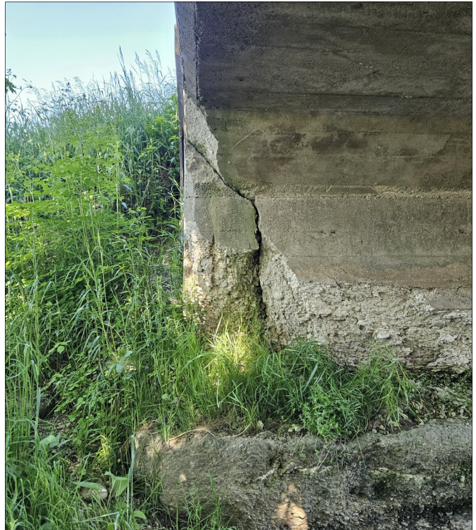
Photo 6 - View of Wide Cracking at Abutment / Wingwall Interface.
