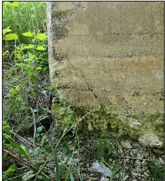
Photo 8 - View of Spalling on East Abutment.
