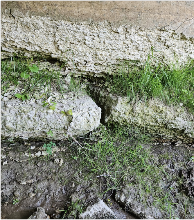
Photo 5 - View of Wide Cracking in West Footing.
