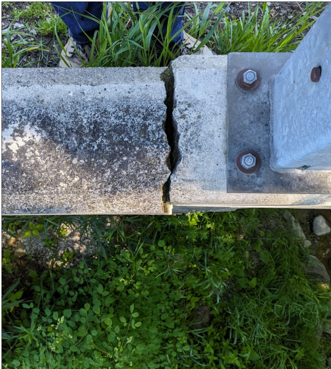
Photo 7 - View of Wide Crack in Curb and Outward Rotation of Wingwall (typ.).
