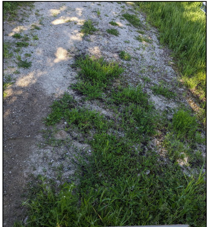
Photo 12 - View of Wearing Surface.
