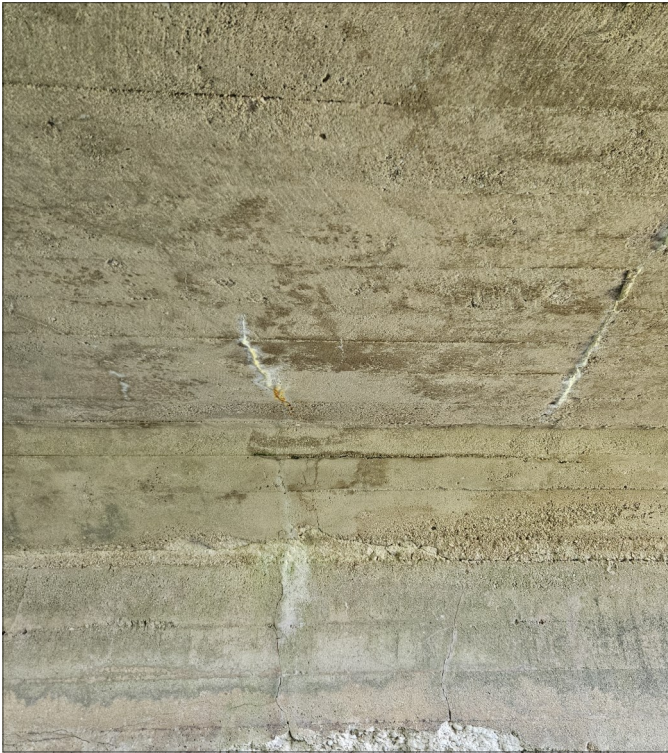
Photo 9 - View of Cracking in the Soffit and Abutment Wall.
