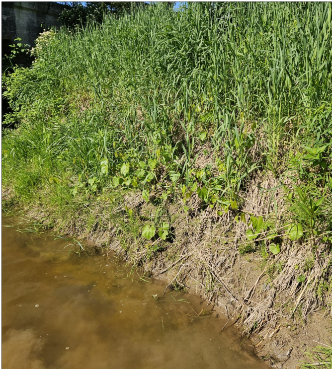
Photo 11 - View of Steep Embankments.
