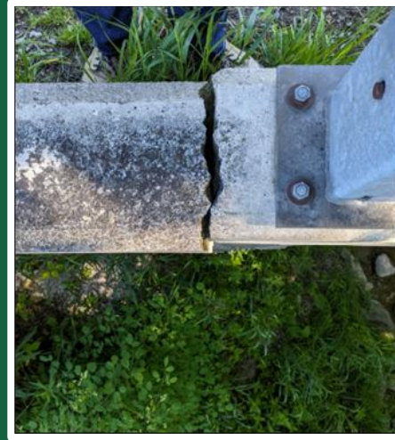
View of Wide Crack & Rotation at Wingwall
