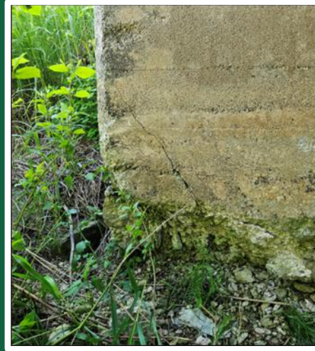
View of Spalling on East Abutment
