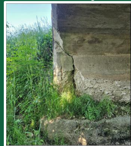
View of Wide Cracking at Abutment/Wingwall
