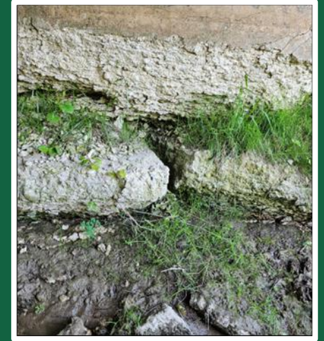
View of Wide Cracking at West Footing
