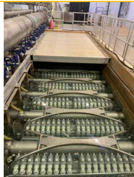
Bare Point Water Treatment Plant filtration system.
